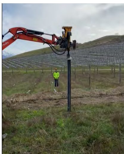
Vibrating digger installing 100% recycled 116mm/2.4m vineyard posts at Cloudy Bay, Central Otago.
